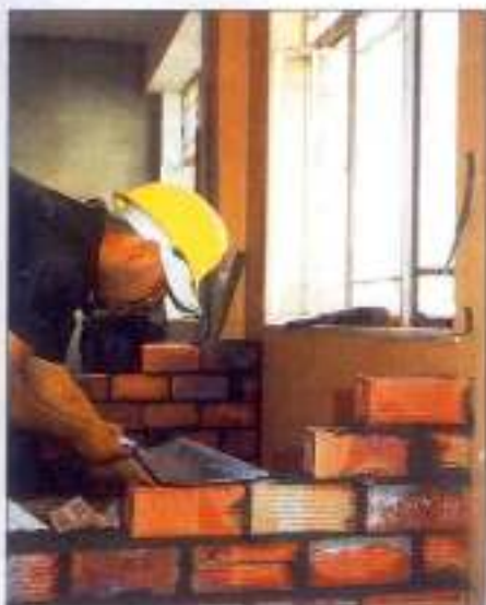
A builder demonstrates the speed and ease of use when using Crammix' new MaxiLite brick for internal partitioning walling
